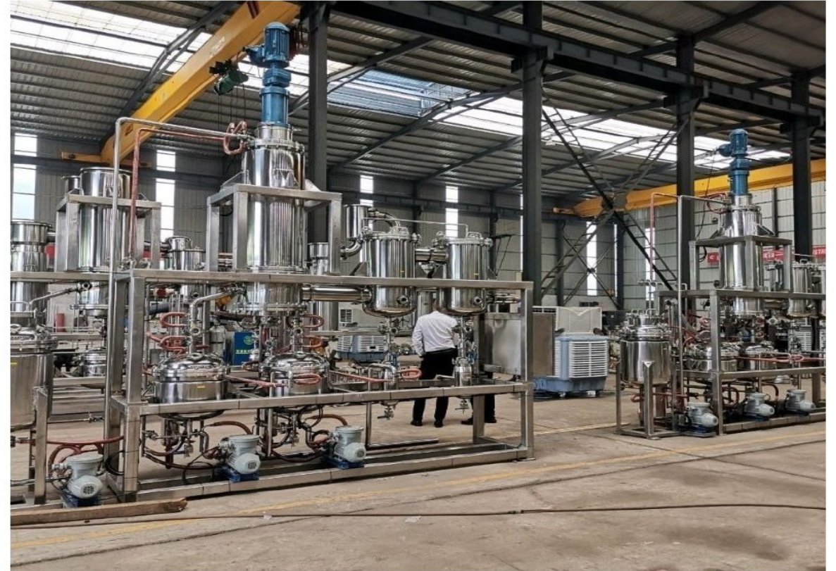
Representative skid-mounted process equipment
